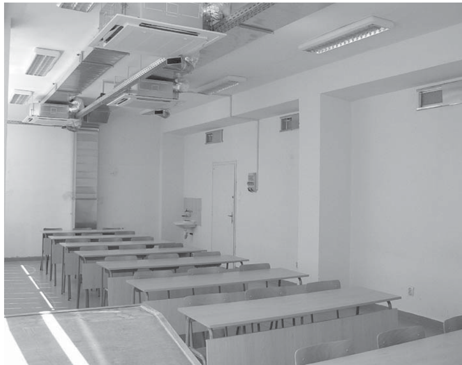
Fig. 9. Right side view of the established laboratory with the installed equipment
